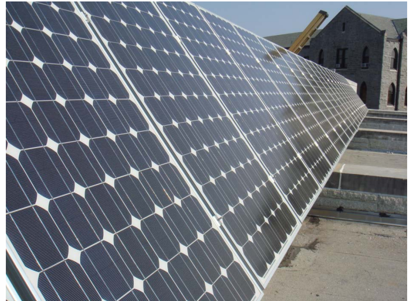
Solar Panels on CEER
