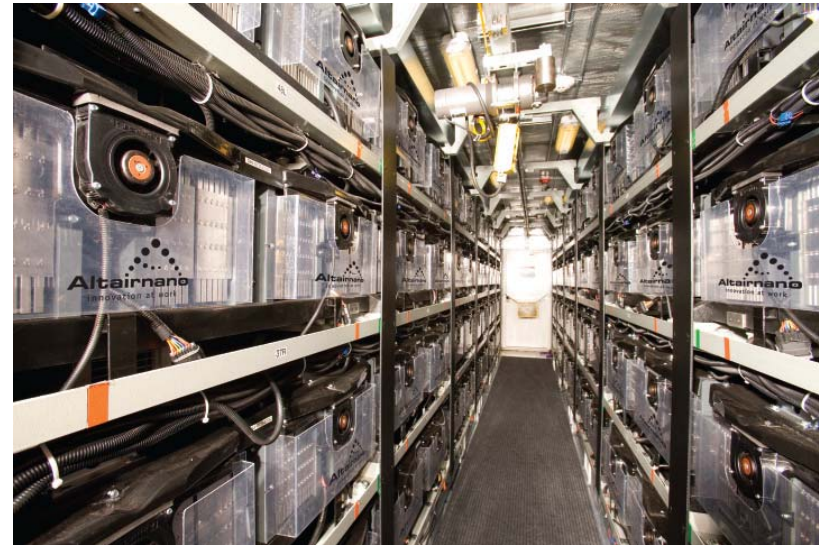
Mobile Utility Battery Storage
